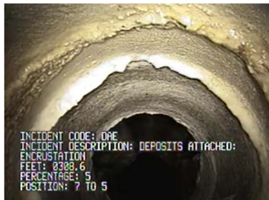
Figure 5 - Deposits Attached: Encrustation.
