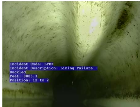
Figure 4 - Lining Failure – Buckled: 12 to 2
